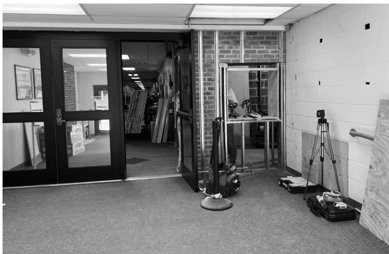
A picture of the new teller-style window under construction in August at the entrance of Iroquois Middle School.
